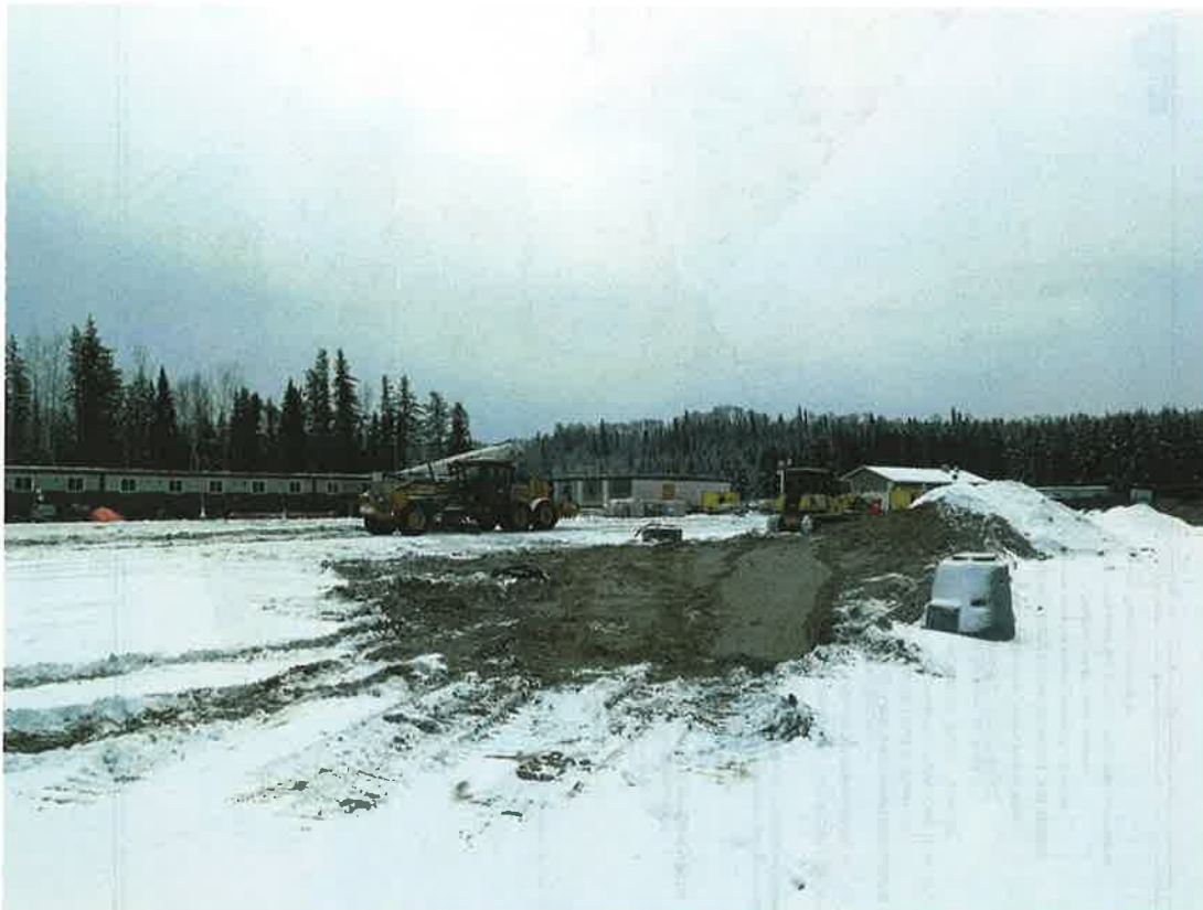
200+ unit dormitory style bunk house and commercial kitchen unit at 15 Goudreau Road.
